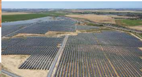
Paymogo Solar Power Plant
