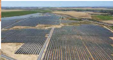
Paymogo Solar Power Plant
